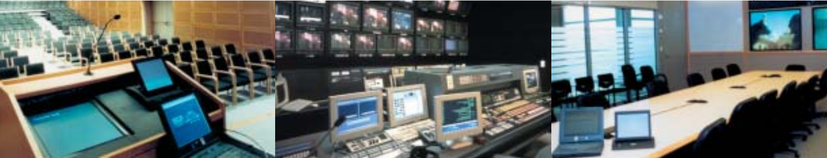
ROSCOR DELIVERS INTEGRATED ELECTRONIC INFORMATION MANAGEMENT SYSTEMS FOR LARGE VENUE LEARNING FACILITIES (LEFT), NETWORK DIGITAL NEWS AND ENTERTAINMENT BROADCASTING (CENTERED) AND SCATTERED CORPORATE TELECONFERENCE CENTERS (RIGHT).
